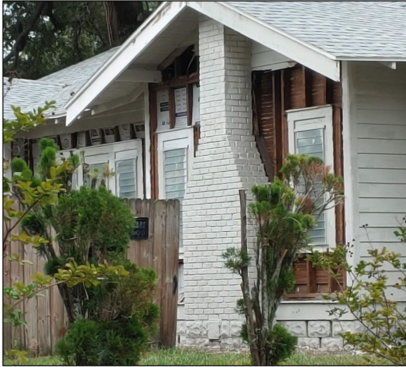
Figure 1: Photograph submitted to the Urban Planning and Historic Preservation Division as part of the neighbor complaint, showing significant siding removal without a building permit or a Certificate of Appropriateness.
